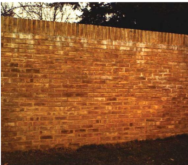
Photo 1 Efflorescence from Water Penetrating Wall Top
